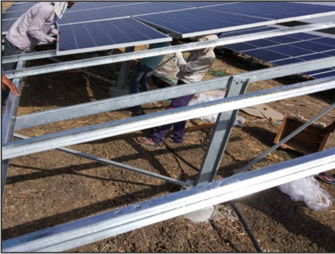
Ground Mounting Structure
